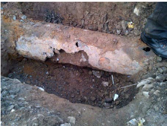
Above: Cambridge Street pipe crossing sinkhole
